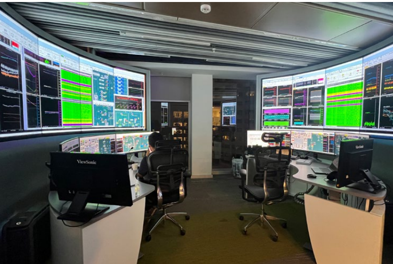
Remote Operation Control Center
