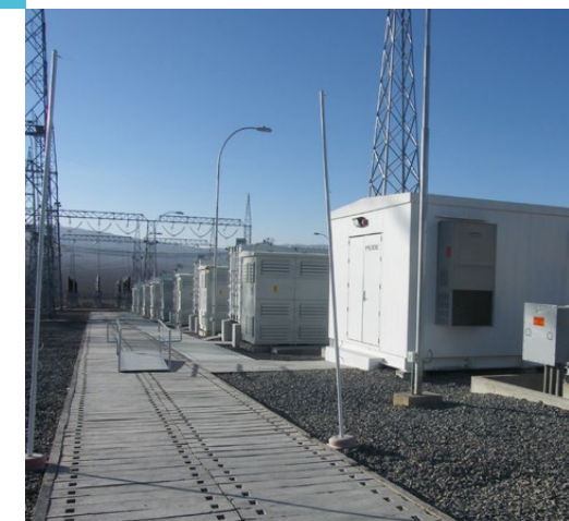
Battery Energy Storage
